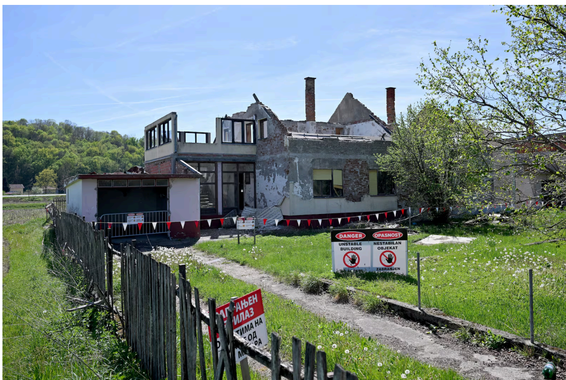
Partially demolished houses bought by Rio Tinto company in the western Serbian village of Gornje Nedeljice. Photograph: Andrej Isakovic/AFP via Getty Images
